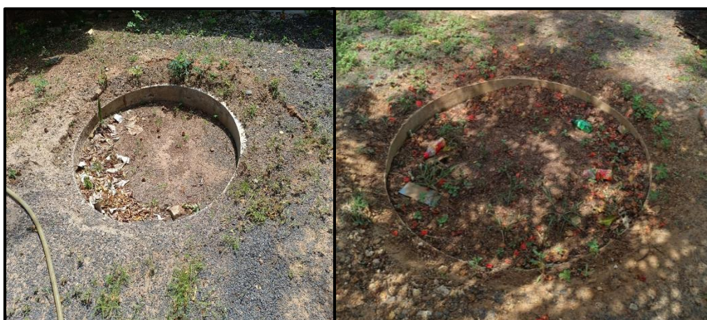
Rainwater Harvesting Activities in St. Ann's college for women, Guntur, Andhra Pradesh.
